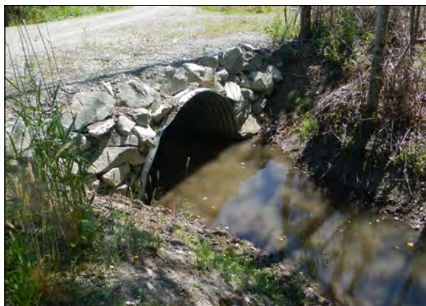
A recently-repaired fish passage culvert. This was originally a 2-foot wide culvert that was routinely plugged by beavers, and is now 11-feet wide.
