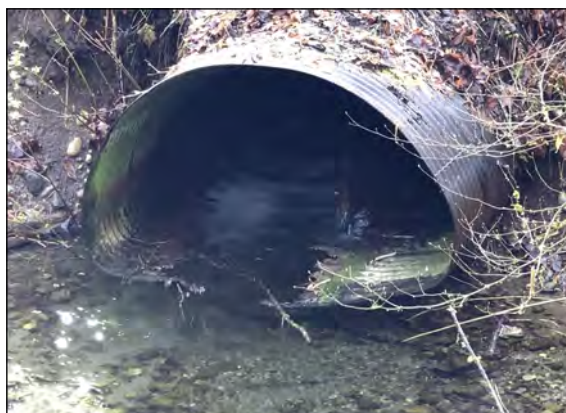
Example of undersized, perched, and failing culvert blocking fish passage while increasing erosion. This culvert is slated for replacement in 2019.
